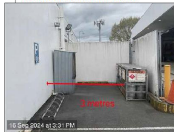
PICTURE 4: ZONE 2 180KG LPG CYLINDER STORAGE CAGE AS SHOWING 3 METERS TO THE MAIN BUILDING EXTERIOR WALL
